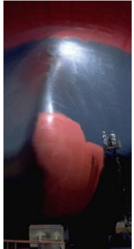
Anti-fouling paint is applied to a ship's hull. (Photograph courtesy Hempel's Marine Paints)
